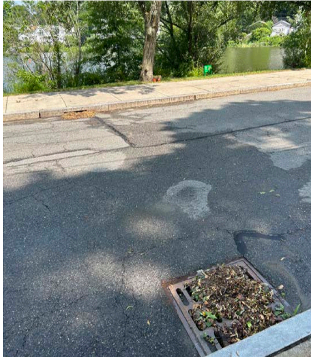
FIGURE 2.9 CATCH BASINS ON LAKE SHORE ROAD This pair of catch basins drains water from Lake Shore Road directly into Chandler Pond.
