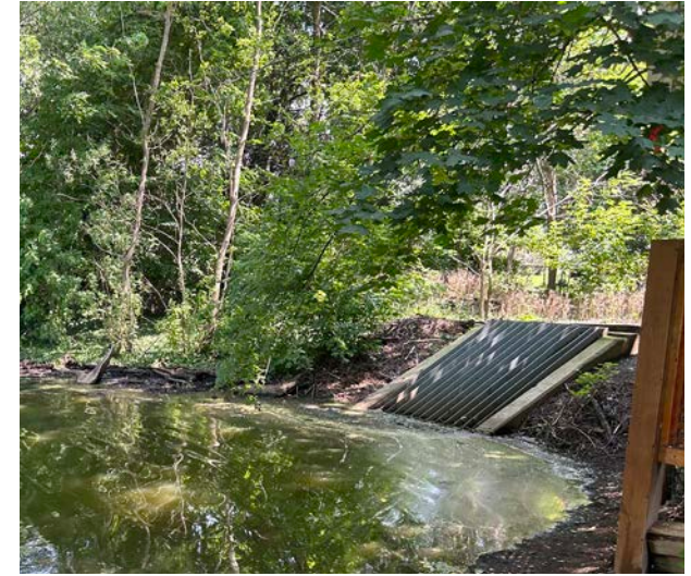
FIGURE 2.11 OUTLET STRUCTURE The pond's single outlet structure is located at the northeast corner of the pond.
